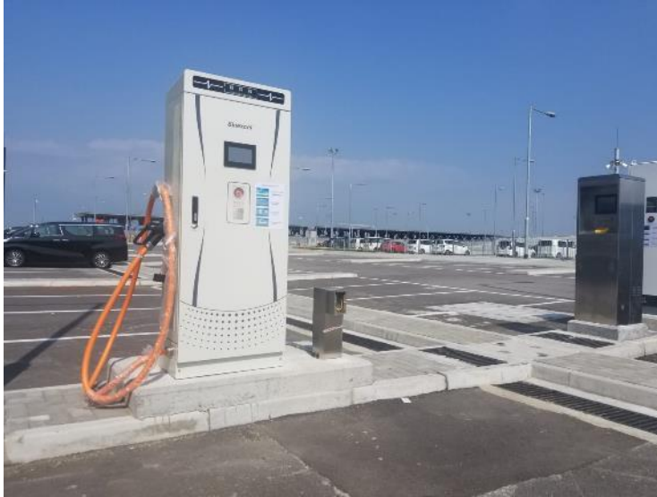
Public Medium & Quick Charging Station at Hong Kong – Zhuhai – Macao Bridge HK Port
